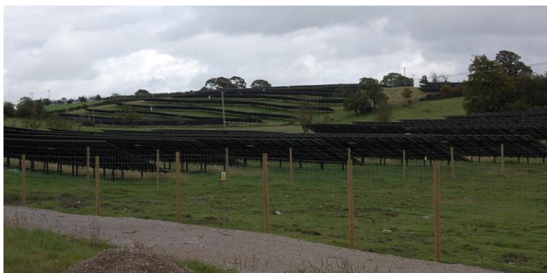
Solar Farm, Ravensclose Road
